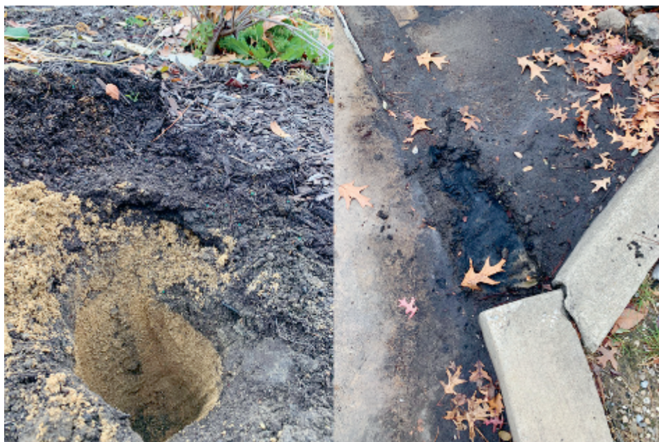
Figure 4. Left picture sampling of filter material consisting of sand with a covering mulch layer at site #22. Right picture a forebay with sediments.
